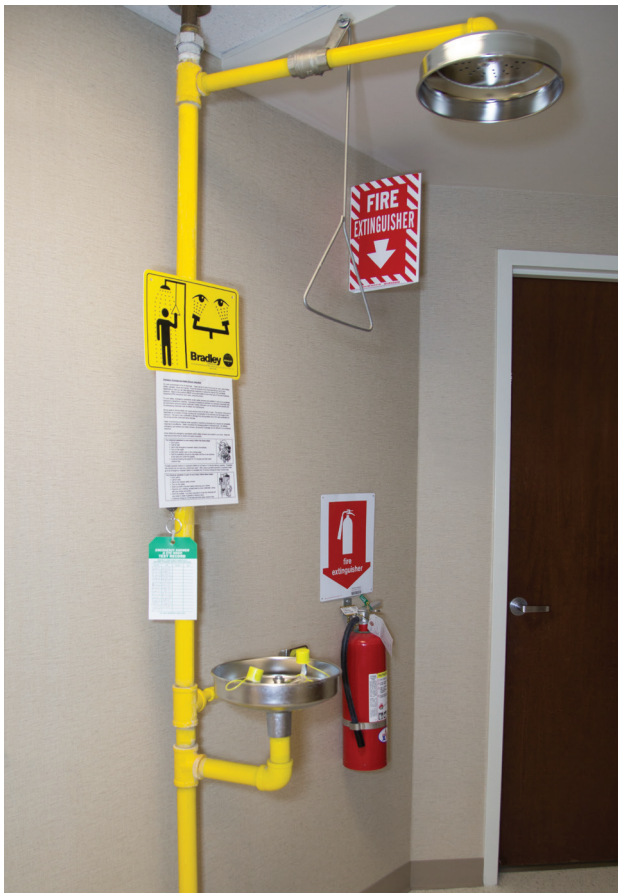
Figure 3-20 Combination safety shower and eyewash.
