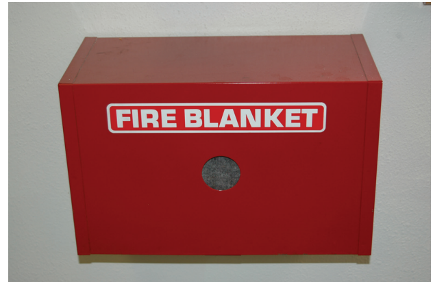
Figure 3-13 Fire blanket storage box.
